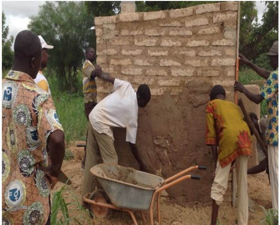
A team of masons building a VIP latrine in the municipality of Komki-Ipala.
